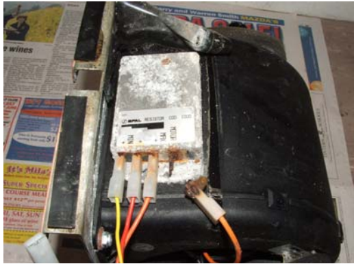
Corroded speed control unit mounted outside
